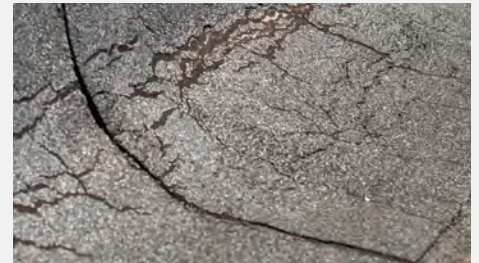
Fix Failing Waterproofing Systems
