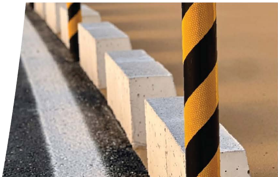
KERB-LINE PROTECTION ON A BRIDGE APPROACH
